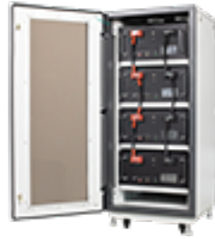
Rack Cabinet Battery
